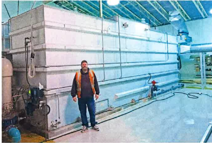
Figure 4: One of the two water trains and our Utility Operator
